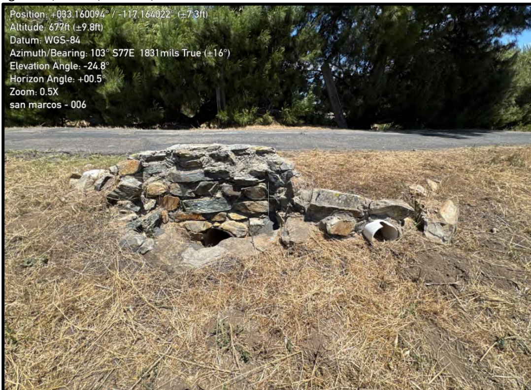
Photo 12: A culvert inlet, located on the eastern boundary of the pond (NWW-S2), runs under the road and installed to manage increased water volume and overflow. There are no hydric indicators east of this culvert and any water flow is considered to be "sheet flow."
