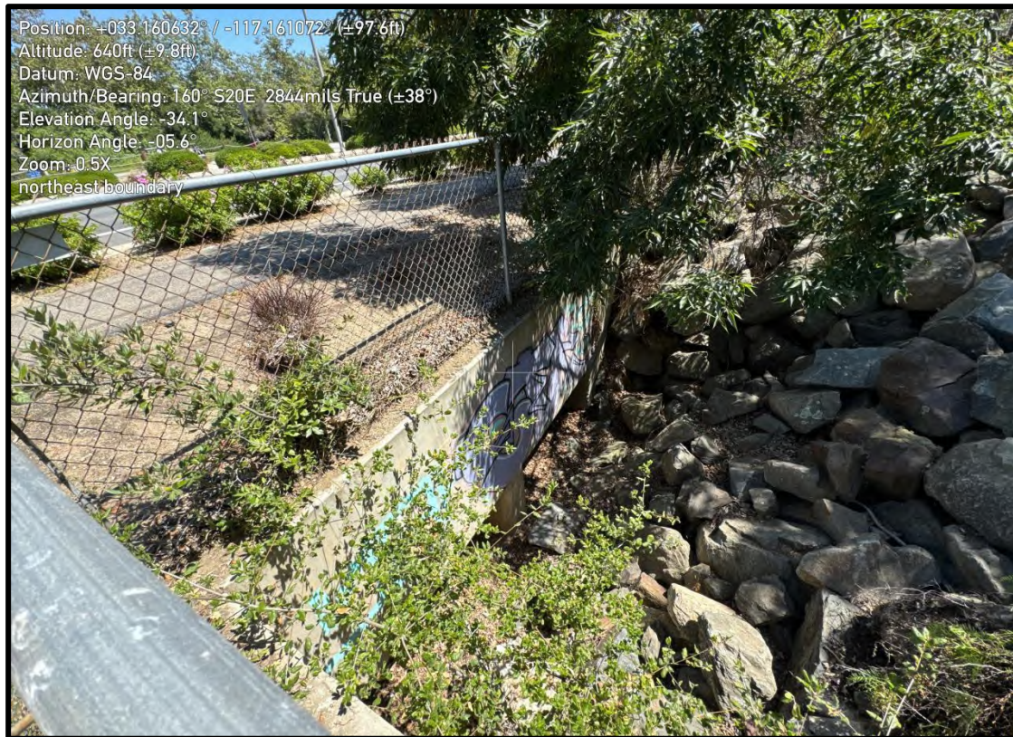
Photo 17: A large, rock lined entrance to a concrete inlet is outside the east boundary of the site to collect any sheet flow coming from the site and channels water eastward under Twin Oaks Valley Road.
